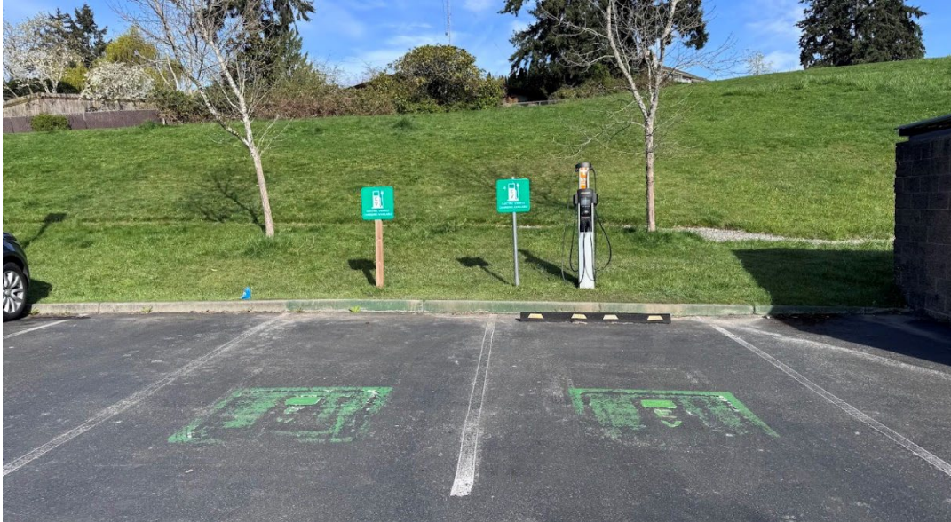
Figure 16: Existing L2 charging ports at MICEC.
